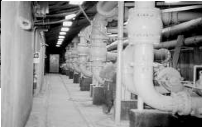
Underground pumping station at the Friedensville Mine, ca. 1976. (Courtesy of Ken Cox.)
