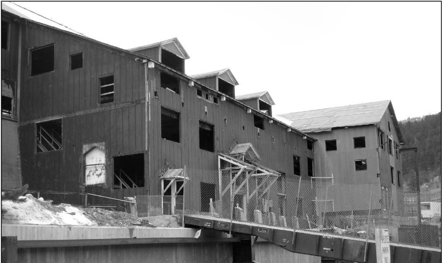
The 1906 Homestake Slime Plant is the last vestige of Deadwood's mining past, and is currently being converted into a casino. (Photo by David Wolff)
